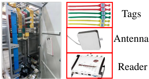
Figure 6: Experimental setup. Include Electrical Cabinet, Reader, Tags, Antenna
